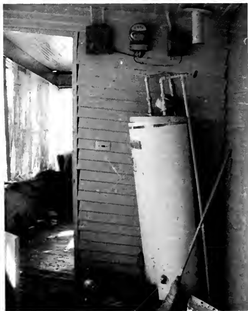
Photo 9. Frame distortion and interior damage in two-story wood-frame house on Orange Grove Avenue, San Fernando, within fault zone. Foundations moved considerably, but no injuries resulted.
